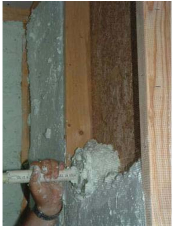
This is a photo of Air Krete ( http://www.airkrete.net ) being foamed into a stud cavity. Air Krete is a magnesium oxychloride-based insulation commercially available since 1984. MPCs and geopolymers can be foamed in several ways suggesting a range of possible uses including stronger and more adhesive insulations.
