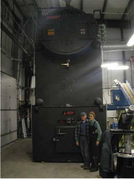
Figure 3: A biomass boiler has been installed to heat the Tok School. Photo courtesy of Alaska Gateway School District.
